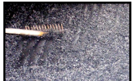
Two mattresses joined together. All gaps are filled with loose rubber crumb from cutting up cells of a mattress.
